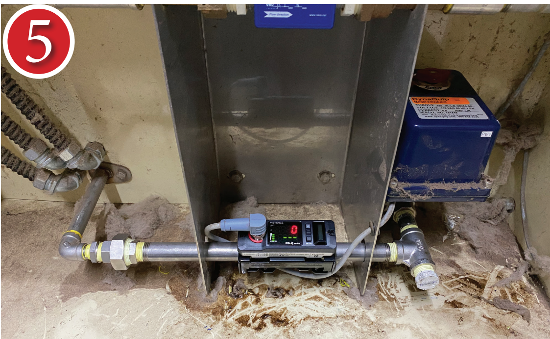
Install new pipe and Clamp-on Flow Meter as pictured. Connect existing cable to meter face.
