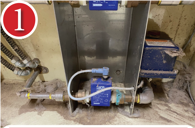
Purge flow meter is on bottom
